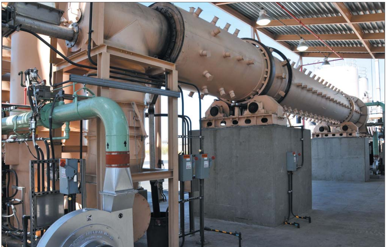
Rotary kiln GAC regeneration furnace at City of Phoenix Lake Pleasant Water Treatment Plant.
