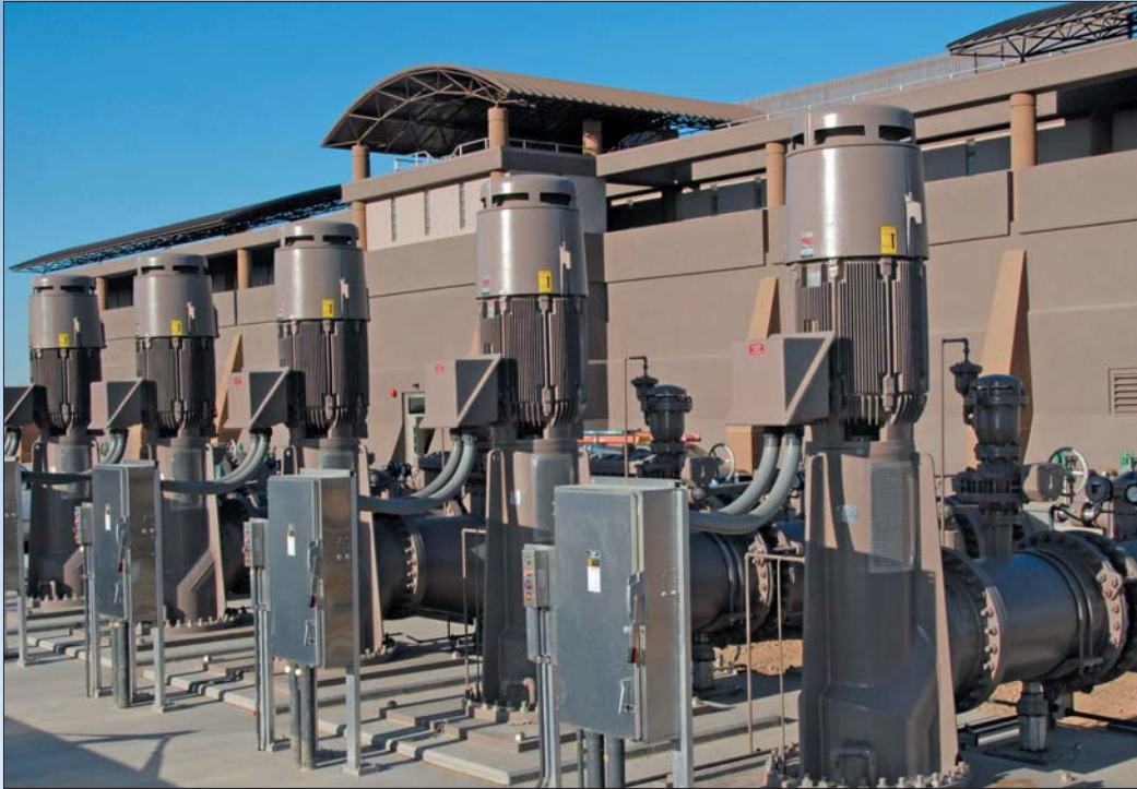
Pump station in front of GAC treatment plant at City of Scottsdale Central Arizona Project (CAP) Water Treatment Plant.
