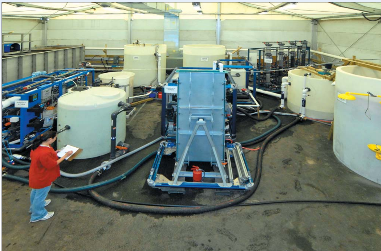
Pilot study facilities for City of Baltimore Fullerton Water Treatment Plant design criteria.
