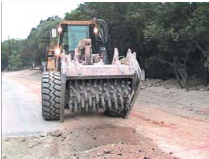
A reclaimer pulverized old asphalt and/or base materials depending on the reclamation depth.
