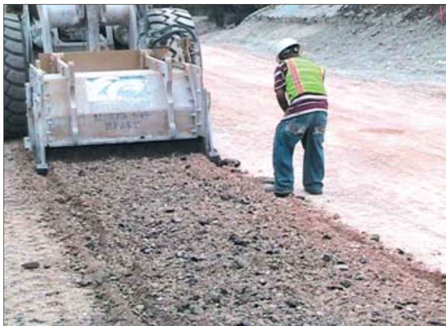
Prior to compaction by rolling, pavement, asphalt, flexible base, and in some areas chip seal material, was pulverized, shaped, and mixed with cement.
