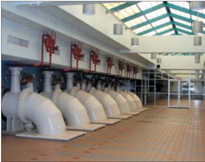
Gallery level in the GCWW GAC contactor building.
