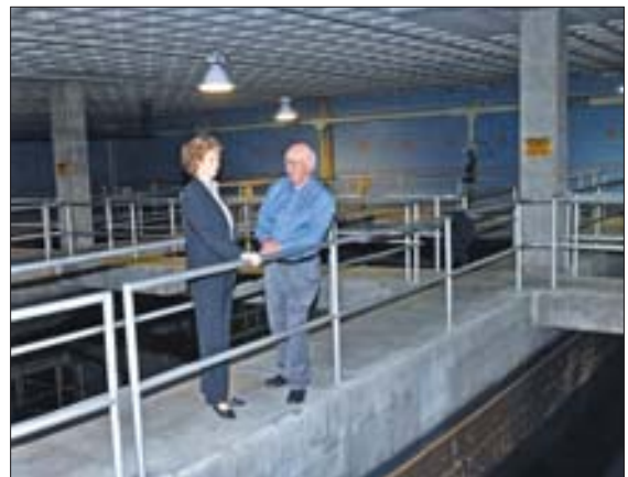
Kristen Atha and Gary Westerhoff at the operating level of the GCWW GAC contactors.
