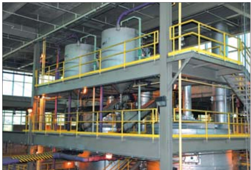
GCWW GAC multiple-hearth regeneration system in the GAC building.
