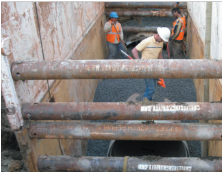
The crushed granite used for backfill covered up to 70 percent of the OD on the shallower depths. For the deeper covers of more than 15 ft, crews placed the same material 12 in. over the top of the pipe.
