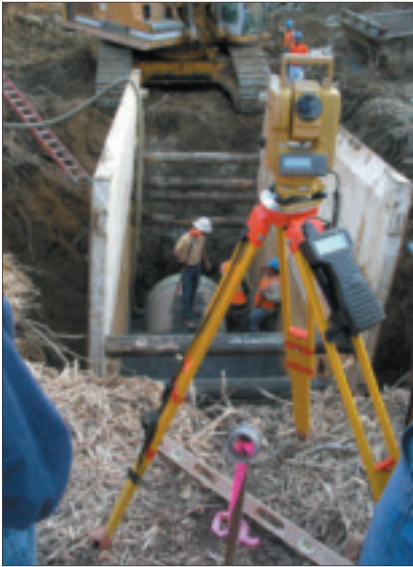
A surveyor's total station is used to direct the location of pipe in the trench during the construction of Deep River Outfall Segment 2 in High Point, NC.
